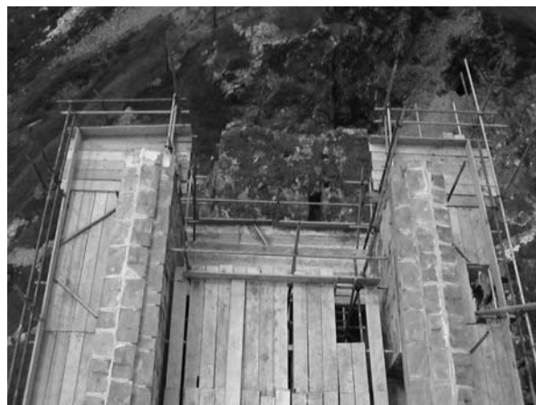
View looking down on slate weathering capping on both wing walls. July 2003. Photo: John Morris
