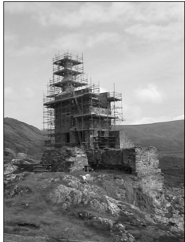
General view of the man Engine House, fully scaffolded , July 2003 Photo: John Morris
