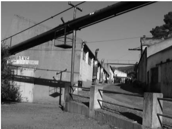
Derelict mill complex, for which there are plans to create a mine heritage centre; or to consider for adaptive reuse.
