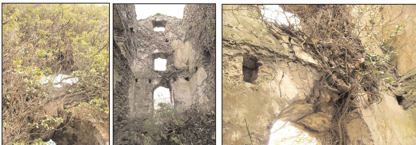
Figure 34. Exterior (left) and interior views of the gable elevation before commencement of conservation works. Ivy growing through and rooted into masonry and brickwork had very severely damaged sections of this wall, especially the lowest arch (right) and all arches had to be extensively reconstructed. This included insertion of stainless steel stabilising pins within wall sections.
